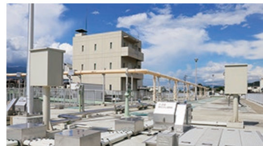
Nagano Prefecture, Iida City Matsuo Purification Center
