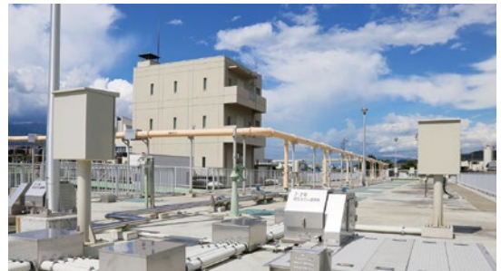
Nagano Prefecture, Iida City, Matsuo Purification Center
