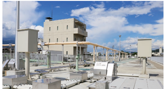
Nagano Prefecture, Iida City, Matsuo Purification Center
